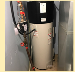
Heat pump water heater
