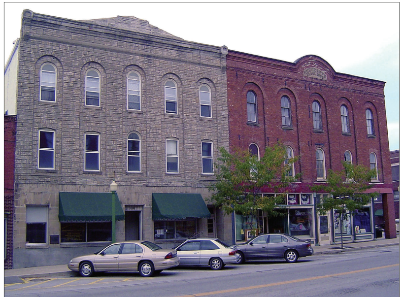
Figure 23. Commercial building with inappropriate synthetic stone on brick facade
